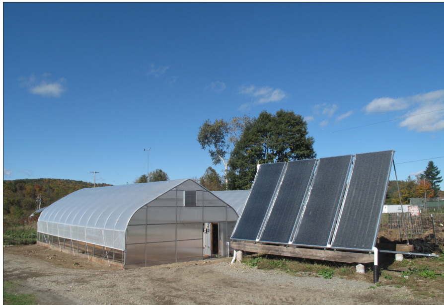
Solar thermal high tunnel system at GMC.
